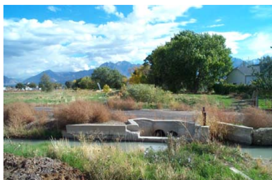
Overflow Structure: North Jordan Canal at Bingham Creek
