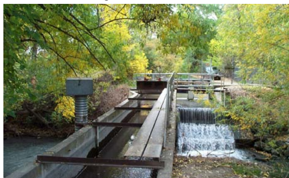
Exchange and Overflow Structure: Jordan and Salt Lake Canal at Big Cottonwood Creek
