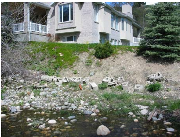
A Deficient Reach along Little Willow Creek, Lower Willow Creek Sub-Watershed
