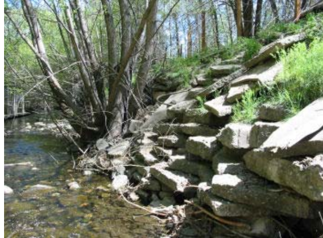
Stabilization structure on Little Cottonwood Creek, Lower Little Cottonwood Creek Sub-Watershed
