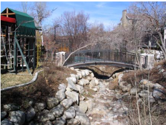
Encroached riparian area, Lower Willow Creek Sub-Watershed
