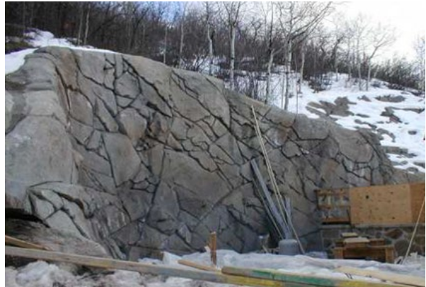
Figure 7. Example of a Soil Nail Wall (Under Construction) with Sculpted Shotcrete Facing
