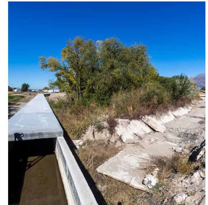
Canal infrastructure replacement reduces water loss to evaporation. Image Credit: Brian Nicholson.
