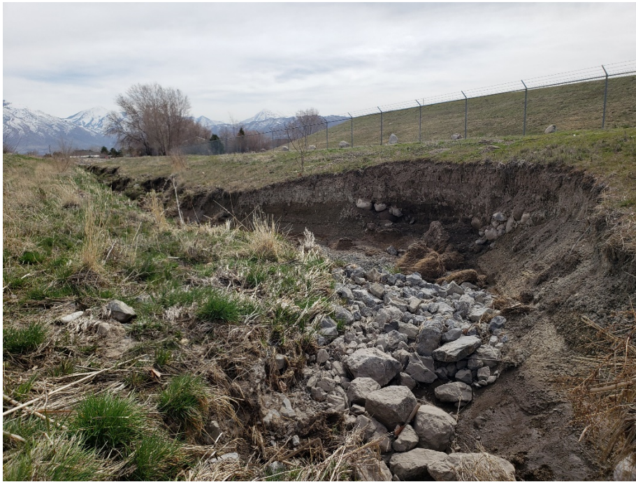
Photo 2-4 Eroded Banks on Rose Creek at approximately 3250 West
