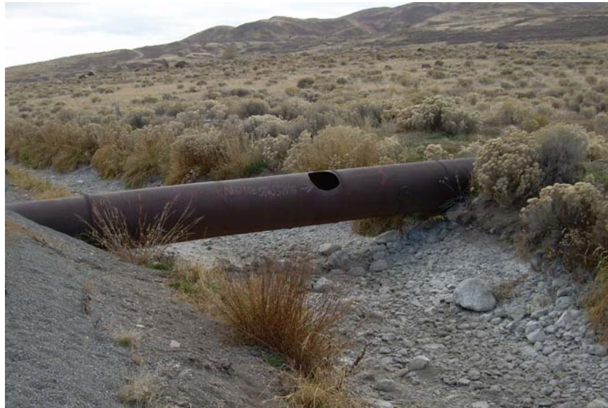
Figure 9. Steel pipe intended to convey substantial Wood Hollow drainage flows across the Provo-Reservoir canal.
