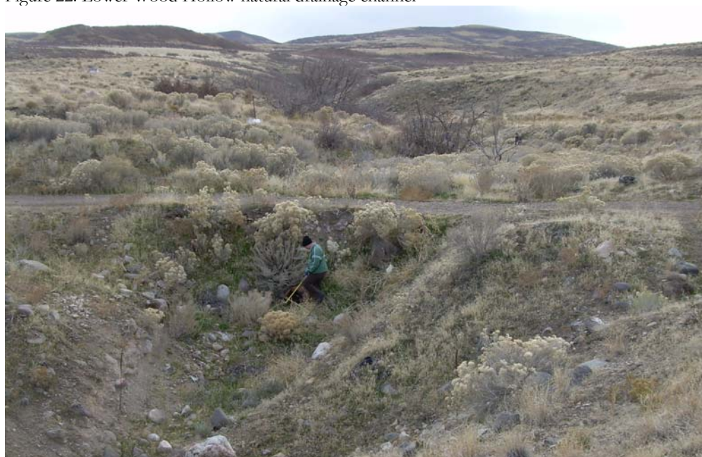
Figure 23. Service road blockage of Wood Hollow's natural drainage channel
