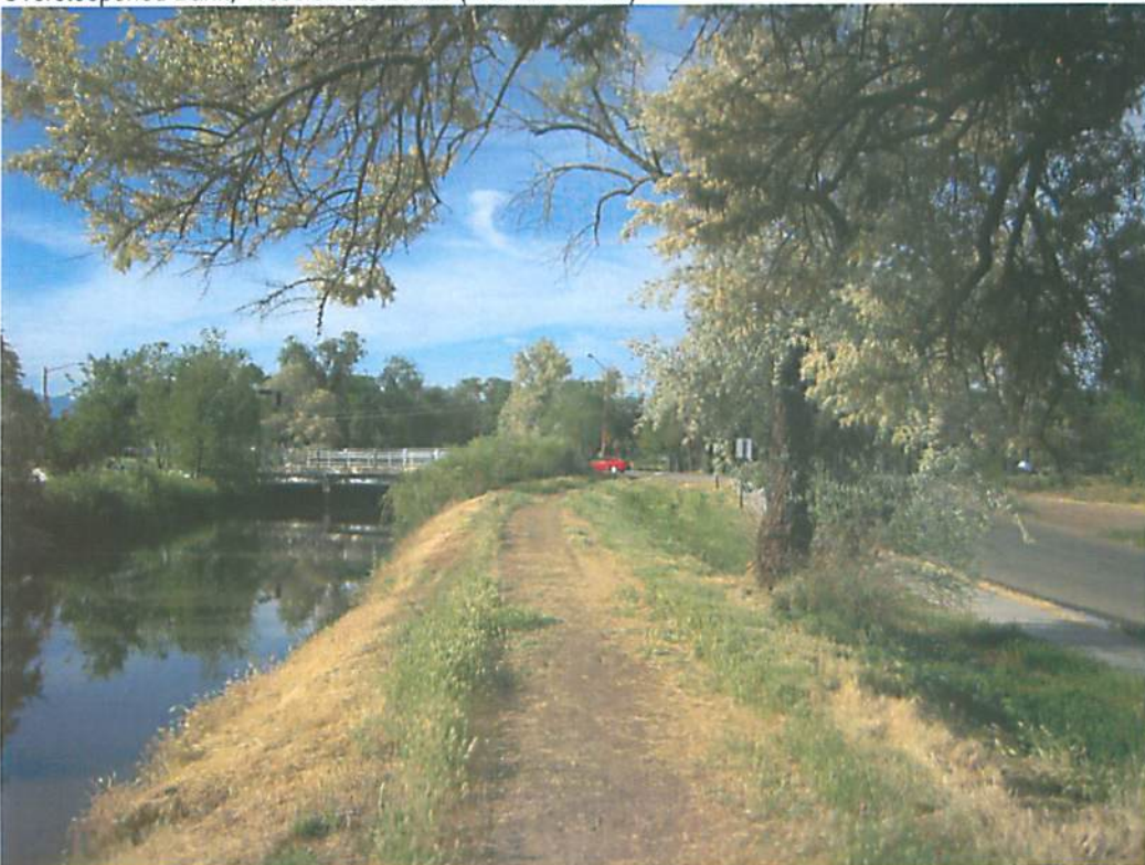
PHOTO 8 Oversteepened Bank, Trees on the Levee (river on the left)
