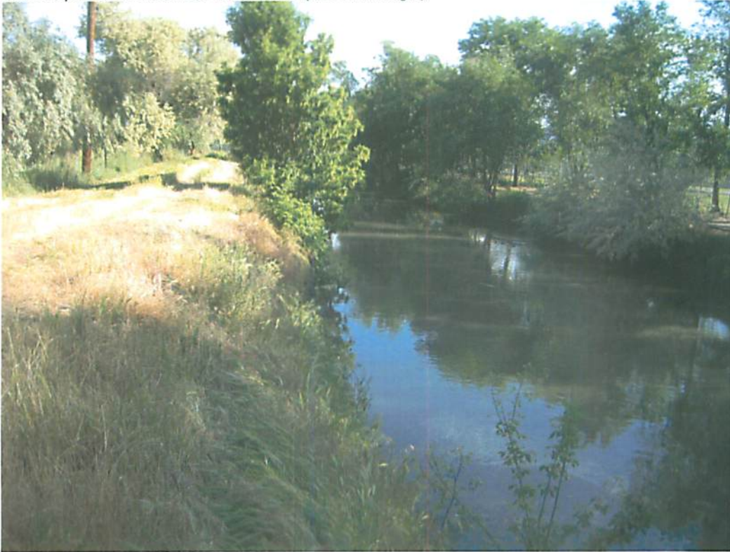
PHOTO 14 Oversteepened River Bank at Toe of Levee (river on the right)
