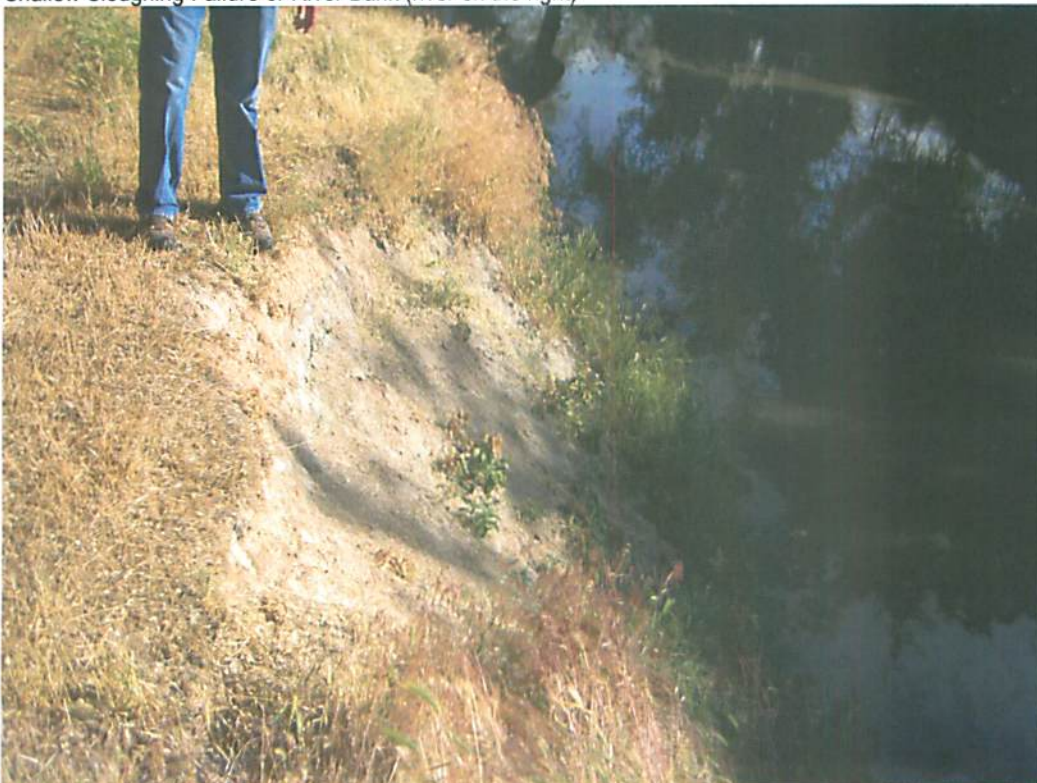
PHOTO 15 Shallow Sloughing Failure or River Bank (river on the right)
