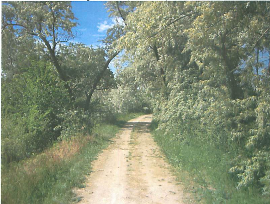
PHOTO 4 Dirt Road on Crest, Trees Growing on the Levee (river on the left)
