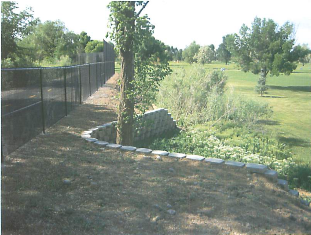
PHOTO 2 Fence, Trees, and Retaining Walls in the, and on the, Levee (river on the left)
