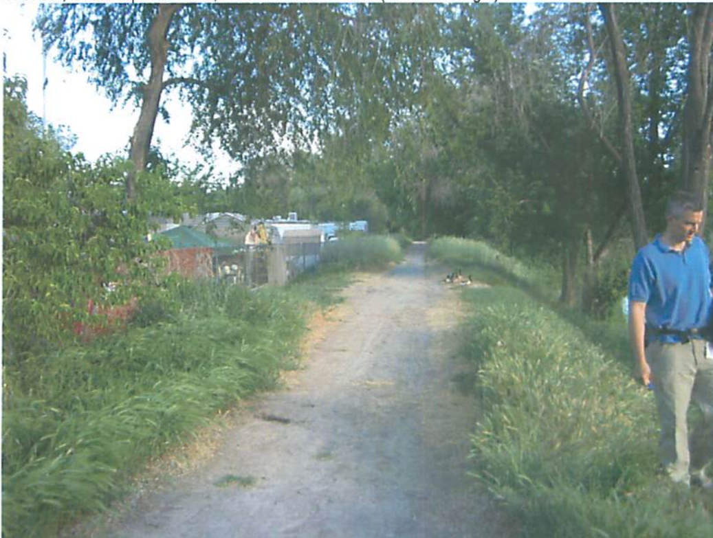
PHOTO 21 Dirt Path, Oversteepened Bank, Trees in Levee Section (river on the right)
