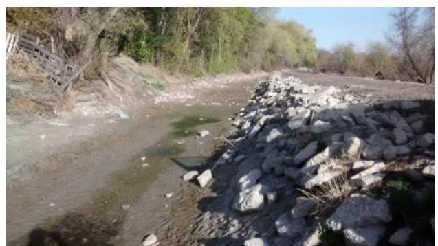
Broken Concrete as Riprap along Embankment – Approximately 8550 South
