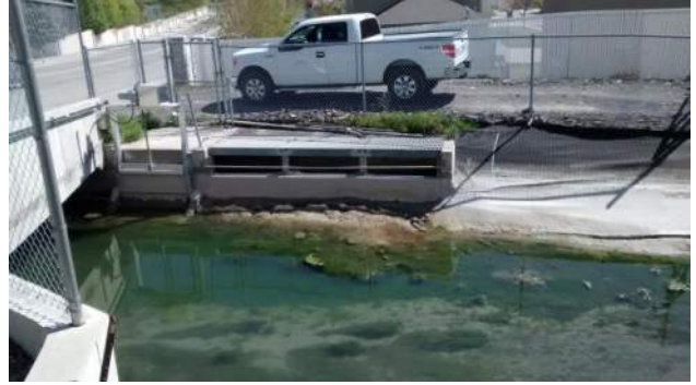
Storm Drain Overflow/Dump-out at Winchester Street
