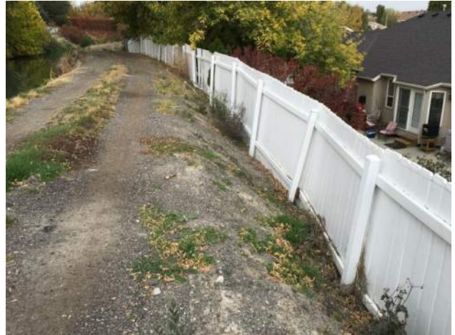
Evidence of Embankment Movement at Approximately 6600 South
