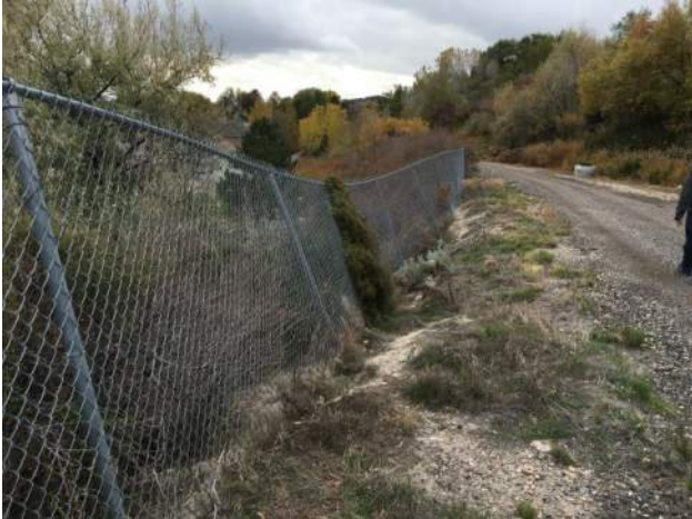
Evidence of Embankment Movement at Approximately 6500 South
