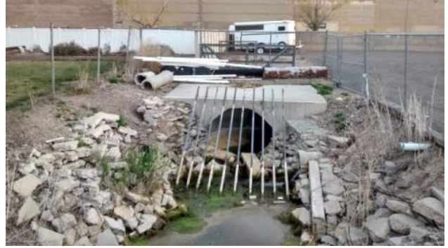
Trash Rack at Approximately 3450 West 3600 South
