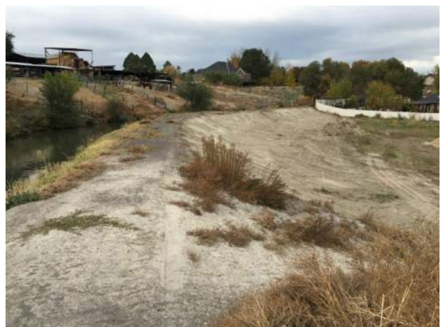
Development Encroachment at Approximately 6400 South
