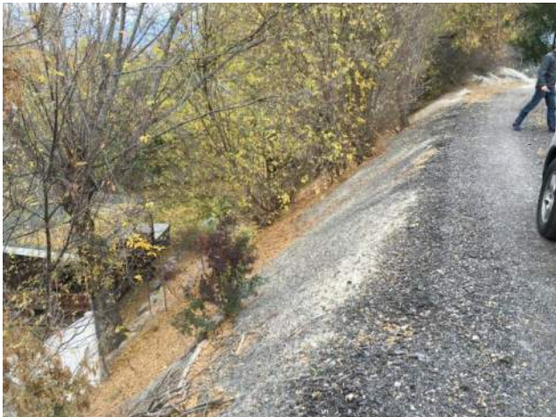
Over Steepened Embankment at Approximately 5500 South
