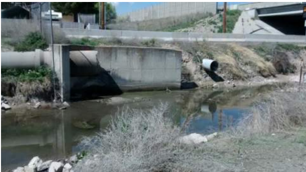
36 inch Pipe outfall at Approximately 5900 South
