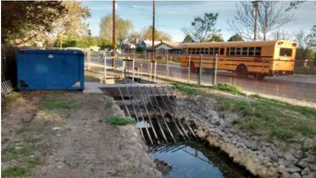
Trash Rack Immediately Upstream of the Outworks to the NJC Pipe
