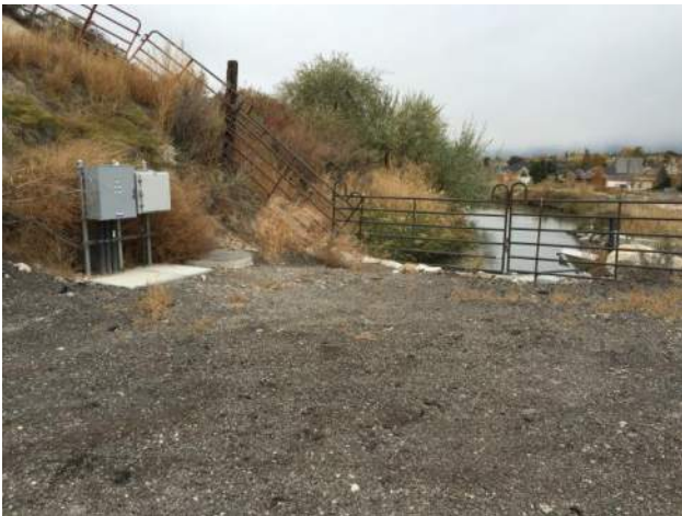
Pump Station on Downstream End of Enclosed Canal Section at Approximately 6450 South
