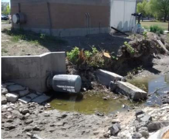
Pump Station Intake at Approximately 2100 West
